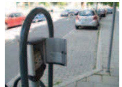
Electric car charging points
